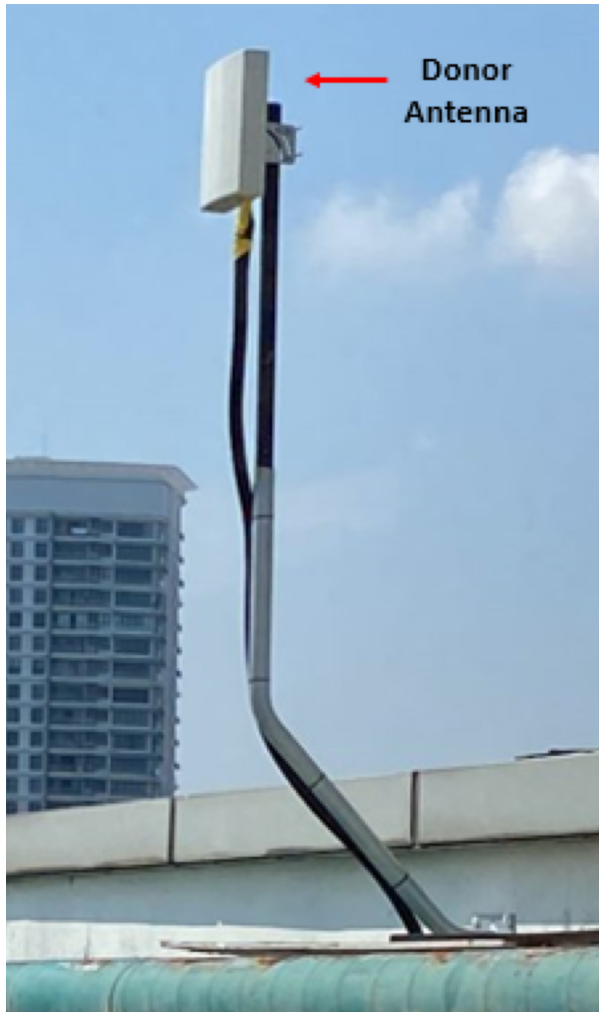
Figure 4: Donor Antenna installed at the rooftop
